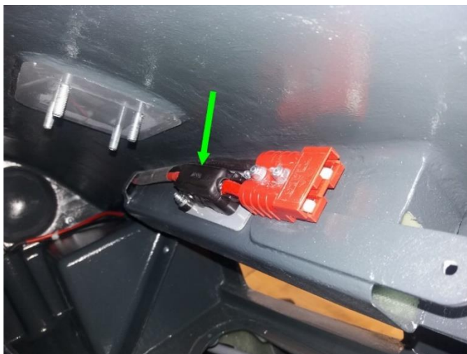
Fig. 2 – Battery connector with fuse box indicated by green arrow.
